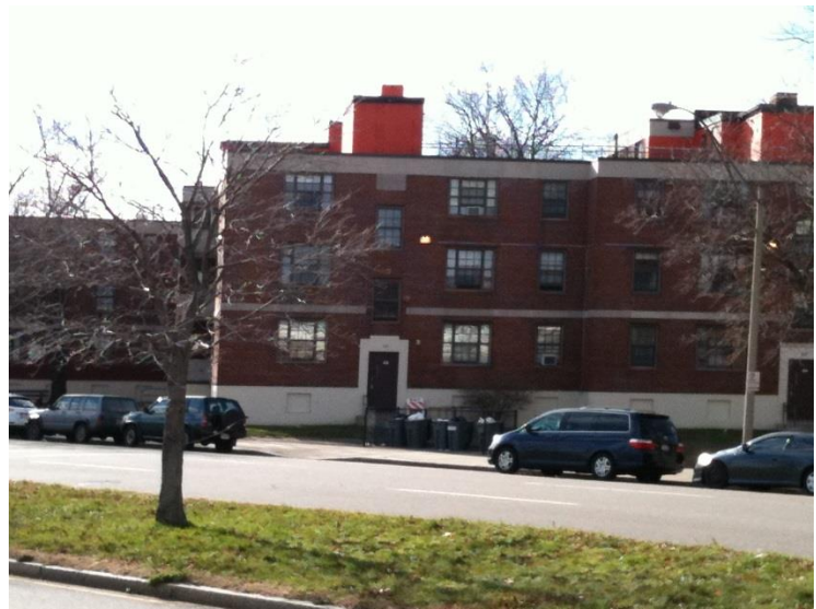
Over 80,000 sq.ft. of WrapShield SA Self-Adhered Water Resistant Vapor Permeable Air Barrier Sheet was installed.
