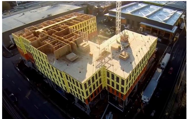
Over 120,000 sq.ft. of WrapShield IT Integrated Tape (orange) was installed over DensGlas ® sheathing.
