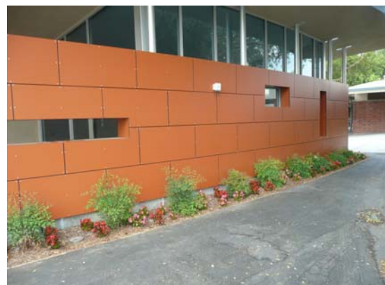
Biola University, Studio B constructed with Trespa panels and WallShield by VaproShield.
