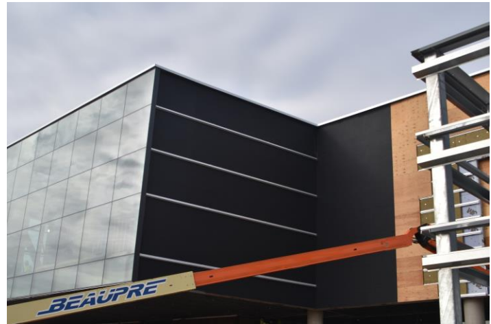
RevealShield SA Self-Adhered (black) was installed on the James Ford Bell Museum and Planetarium facility on the St. Paul campus of University of Minnesota
