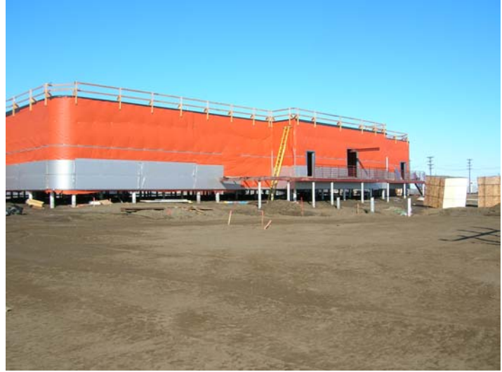
Phase I of NOAA Global Climate Change facility. WrapShield (orange) installation and cladding (silver) in progress. 6/25/06
