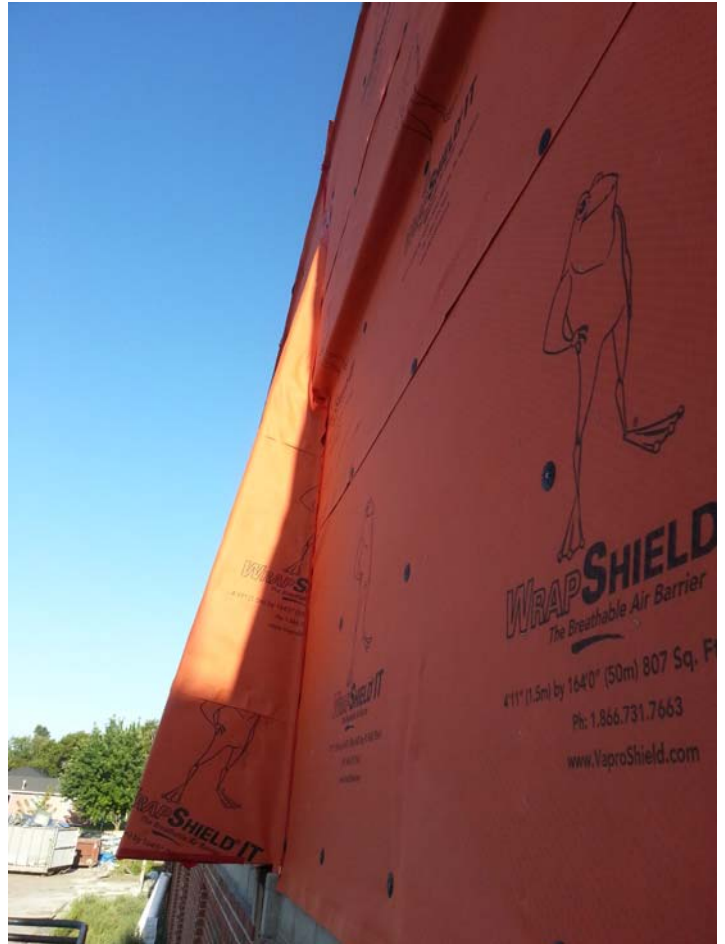
Over 10,000 sq. ft. of WrapShield SA Self-Adhered Air Barrier was installed on Franklin Middle School in Thief River Falls, Minnesota.
