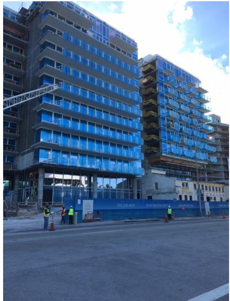
Over 10,000 sq.ft. of WrapShield SA Self-Adhered WRB/Air Barrier was installed on the new additions to the Surf Club Four Seasons in Miami, Florida.
