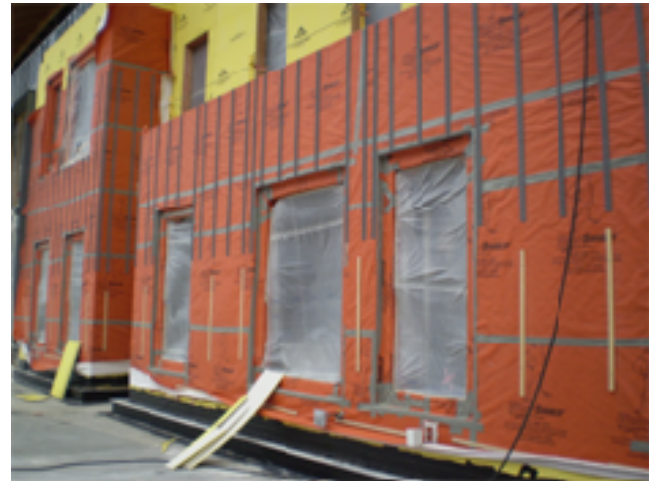
WrapShield combined with VaproBatten and Rain Screen Design Components were used on Epic Corporations Building K.
