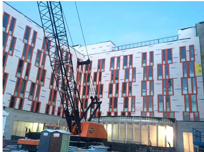
Over 43,000 sq. ft. of WallShield Water Resistive Barrier Sheet is being installed on the ANTHC Patient Housing building in Anchorage.
