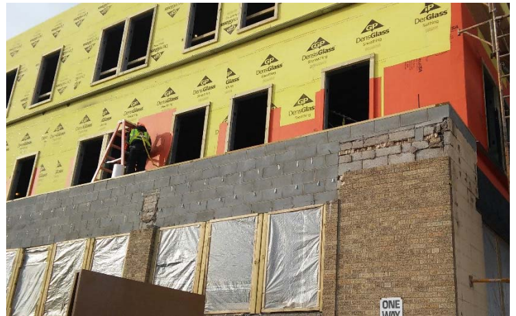
Over 19,000 sq. ft. of WrapShield SA Self-Adhered Water Resistive Vapor Permeable Air Barrier Sheet was installed at 345 State Street Apartments in Grand Rapids, MI.
