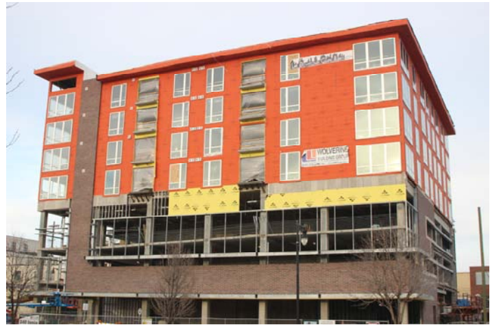
Over 27,000 sq. ft. of WrapShield was installed on 240 Ionia in Grand Rapids, Michigan.
