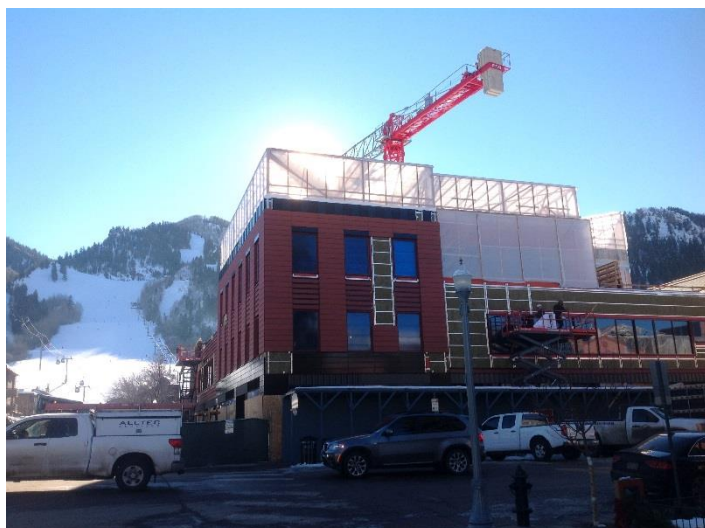
Over 20,000 sq.ft. of WrapShield SA Self-Adhered was installed behind wool insulation and terra cotta on the Aspen Core Penthouse.
