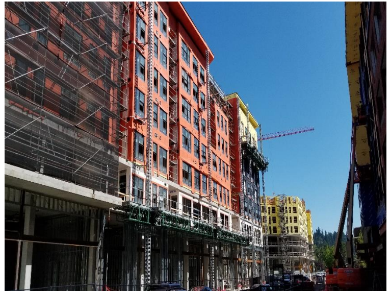
RevealShield SA was used on 10% of this project in areas with open joint siding systems. RevealShield SA will provide long term UV stability from the sun's rays.
