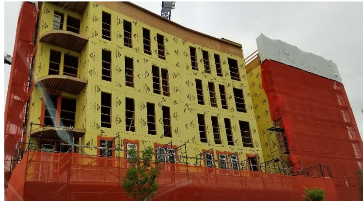
Throughout the building process, over 300,000 square feet of WrapShield IT Water Resistive, Vapor Permeable Air Barrier Sheet is installed over the outer facing of the project.
