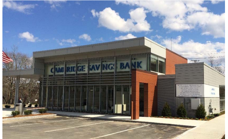
Fundermax exterior panels were installed over RevealShield SA Self-Adhered, creating the desired black open joint reveal.
