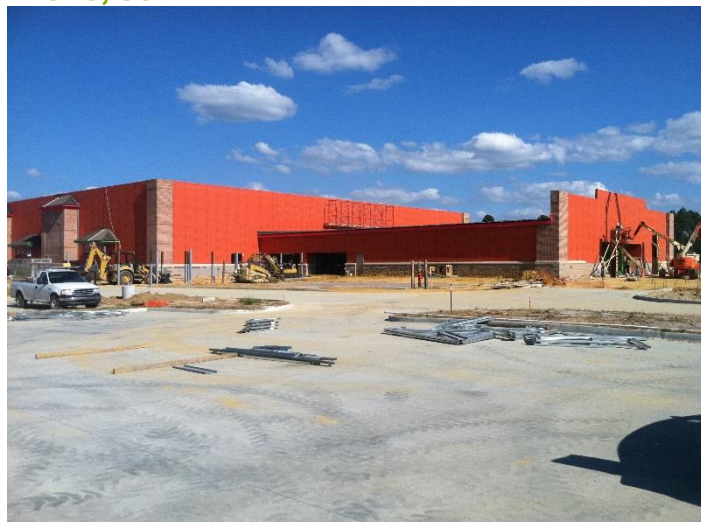
Over 31,500 sq.ft. of WrapShield SA Self-Adhered Water Resistive Vapor Permeable Air Barrier was installed.
