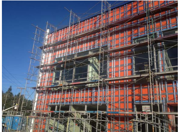
Over 5,000 sq. ft. (464 M 2 ) of WrapShield SA Self-Adhered Air Barrier is installed on the Parker Johnston Ltd. building in Victoria, British Columbia.
