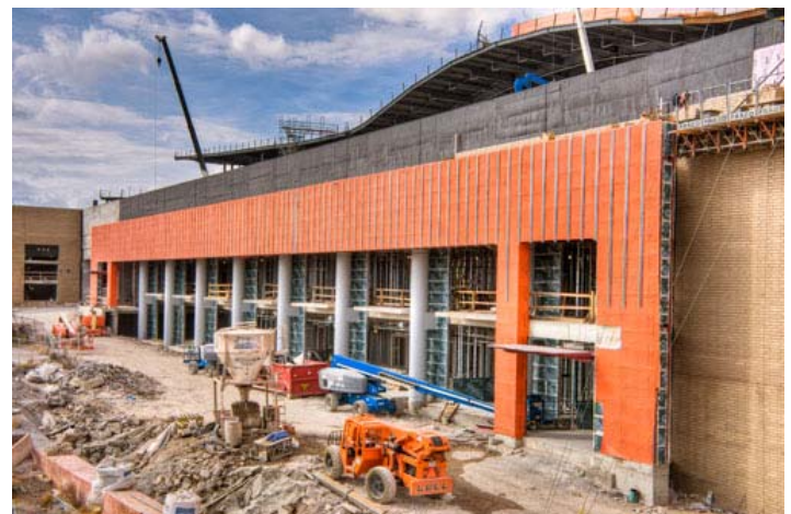
WrapShield SA Self-Adhered (orange) installed as part of a rain screen system, under the battens (gray vertical parts).
