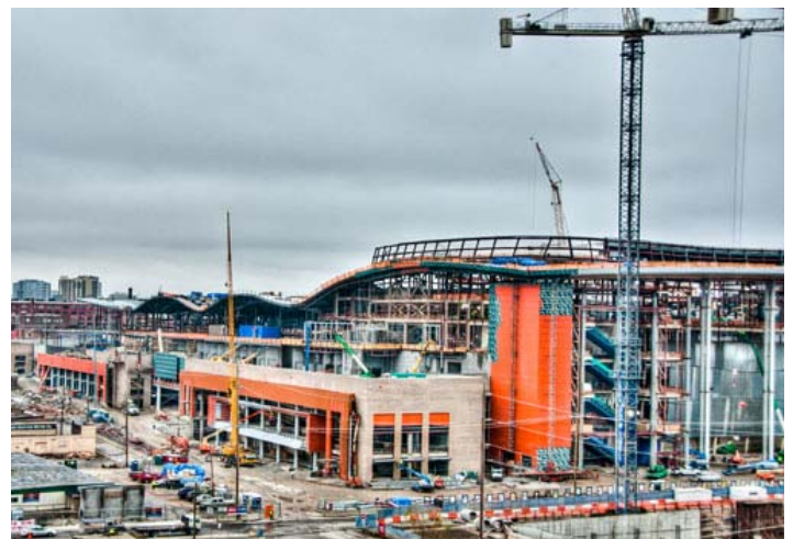
The project totals 16 acres and 2.1 million sq.ft. Over 400,000 sq.ft. of WrapShield SA Self-Adhered was installed over 12 months, with no delays due to weather or special equipment needed onsite.
