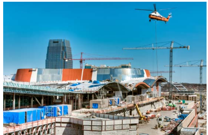
WrapShield SA Self-Adhered was installed over insulation on the guitar-shaped pop-up section of the roof.
