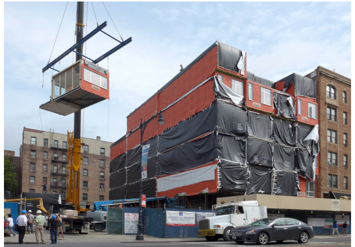
Over 32,000 sq. ft. of WrapShield SA Self-Adhered Water Resistive Vapor Permeable Air Barrier Sheet was used on this modular apartment building.
