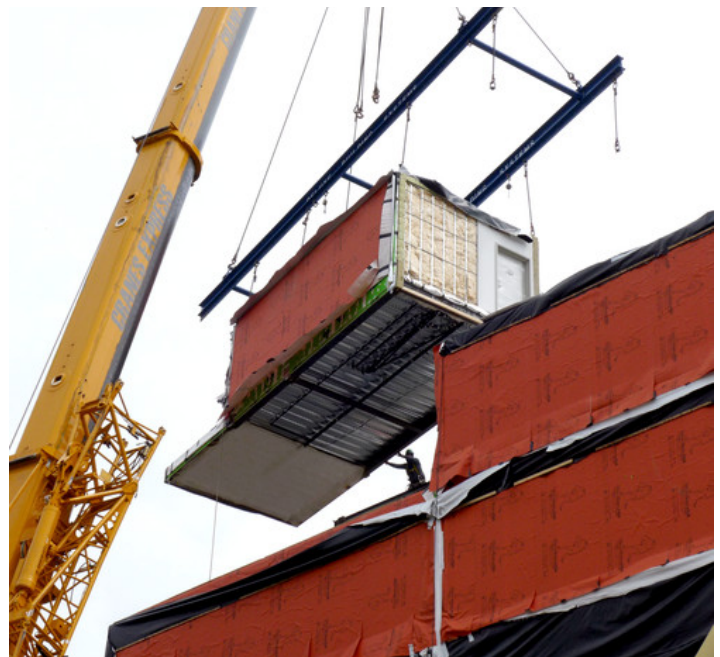
Modular unit being put in place. WrapShield SA Self-Adhered (orange) is on multiple sides of each unit. Photos courtesy of Gluck+.
