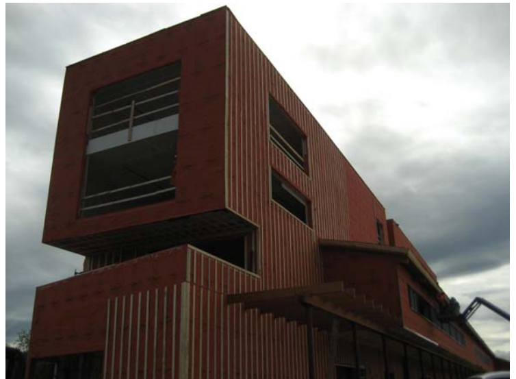
Over 48,000 sq. ft. of WrapShield SA Self-Adhered Water Resistive Vapor Permeable Air Barrier Sheet was installed on the Waterfront Station commercial center in Whitehorse, Yukon. All photos courtesy of Mary Ellen Read.
