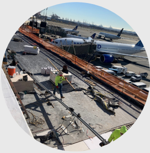
Work continues on reroofing with robust weather protection installed. Building remains occupied.
