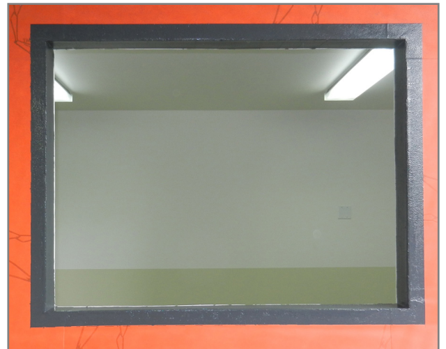
VaproLiqui-Flash is applied inside the rough opening and 1" on the face. The completed rough opening is now ready for window installation.
