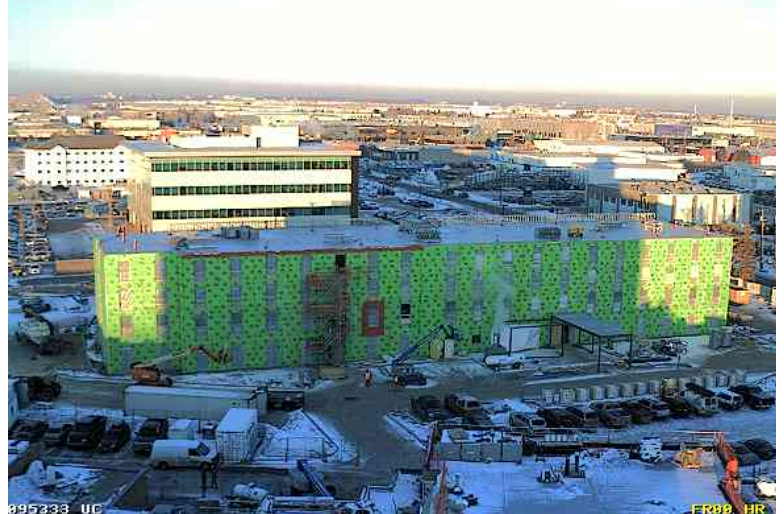
Construction begins on the SilverBirch Hotels & Resorts Home2 Suites in Edmonton, Alberta. WrapShield SA Self-Adhered Air Barrier (orange) is applied over the rough-opening of a second story window. Photo courtesy of: www.silverbirch.com
