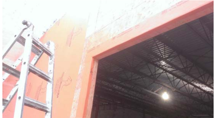
Over 10,500 sq. ft. of WrapShield SA Self-Adhered is installed on the Audi Dealership of Mentor, Ohio.
