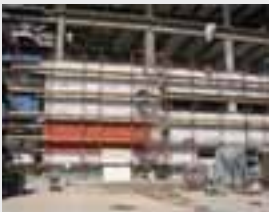
Veterans Administration Healthcare System in North Las Vegas installed 300,000 S/F of WrapShield SA.
