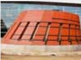
Self-Adhered is featured on "The Grotto," a 9000 S/F addition to Brody Hall at Michigan State University.
