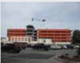
Over 60,000 S/F of WrapShield SA (Self-Adhered) was installed in the $150 million expansion project of the Central Washington Hospital, WA
