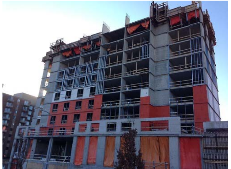
Over 100,000 sq.ft. of WrapShield SA Self-Adhered Water Resistive Vapor Permeable Air Barrier Sheet was installed.
