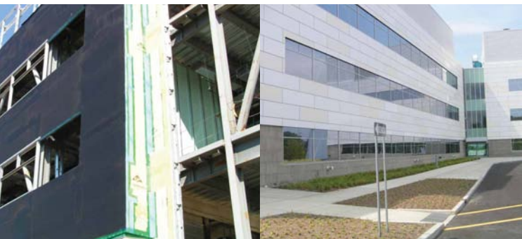
During and after construction shots of the cancer research center at SUNY Albany in Rensselaer, NY, shows a system Air-Bloc 33 permeable, fluid-applied air barrier, UV-resistant coating, and a Trespia, METEON composite panel system outboard air barrier. The architect was Einhorn, Yaffe and Prescott of White Plains, NY, and the air barrier subcontractor was Cornerstone Waterproofing of Cooperstown, NY.
