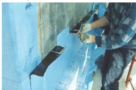
Is sheet the best solution? Sometimes there is difficulty when using a sheet membrane system with pre-installed brick ties and penetrations. Fluid-applied systems can be less costly to install and may produce better results in some cases.
