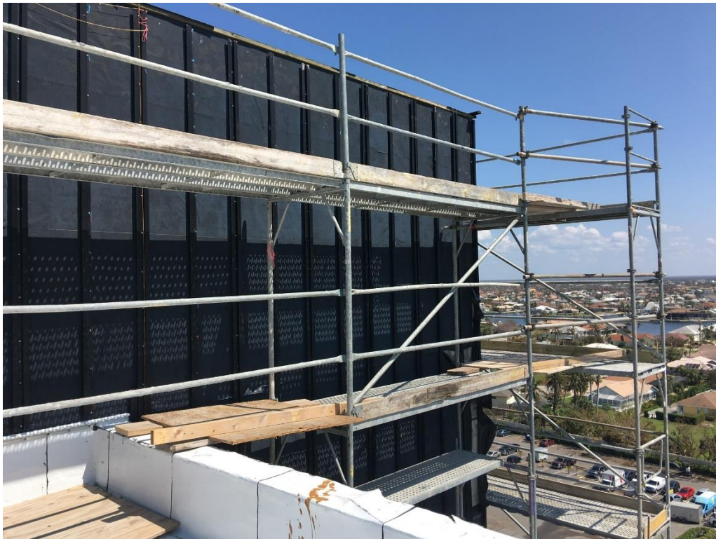
To the relief of installation crews, less than 10% of the membrane was damaged.
