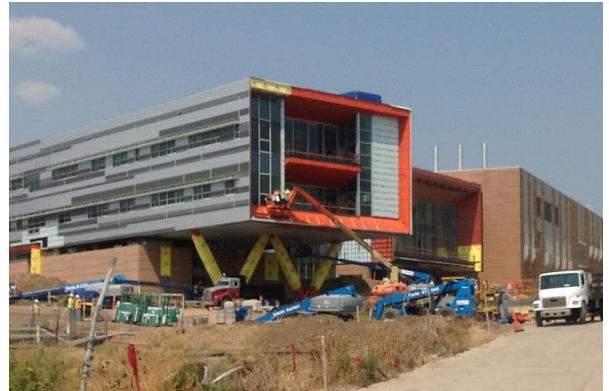
National Renewable Energy Lab , solely dedicated to advancing renewable energy and energy efficiency technology, achieved LEED Platinum status using VaproShield products.
