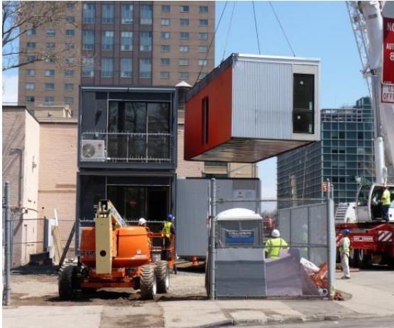
WrapShield SA® Self-Adhered Water Resistive Vapor Permeable Air Barrier Sheet (orange) provides superior protection on NYC's Post Disaster Housing Prototype. Photo courtesy of Mary Frost.
