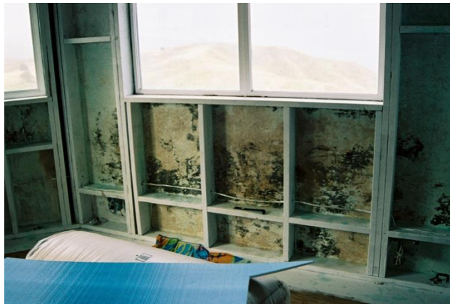
Figure 1: Damage due to limited drying potential.
